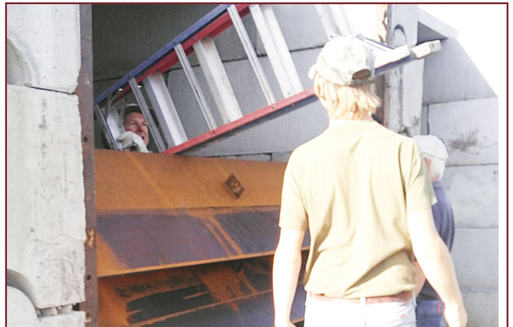
Klay Carver looks on as Mark Jungmann directs the crew in erecting the steel baffles for the new pistol range. Jack Miller constructed the baffles, using new half-inch thick steel plate just purchased, and "steel from an old rod weeder I took apart years ago."
